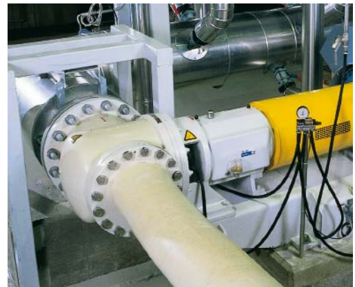
Fig. 2. MC® equipment applications in a modern bleaching plant.
