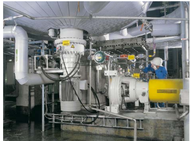
Fig. 17. MC® tower discharge pumping system.
